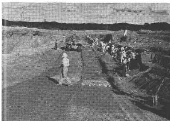
FIG. 11. Prospect pits in residual weathered rock representative of the hundreds of such pits near Sete Lagôas, Minas Gerais. The bedrock in this region is red shale. Rock fragments are bull quartz.
