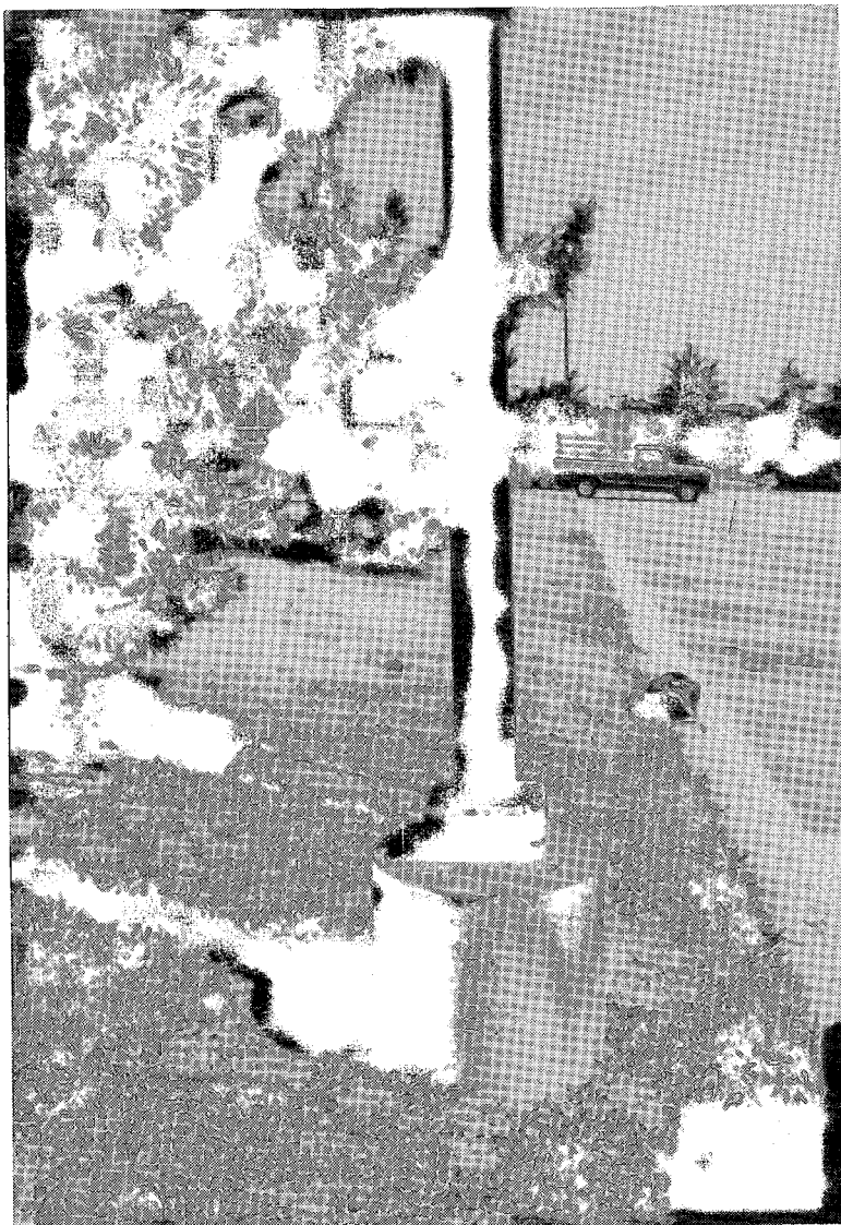
FIG. 8. Staining of concrete by runoff from weathering steel. College Park, Maryland.
