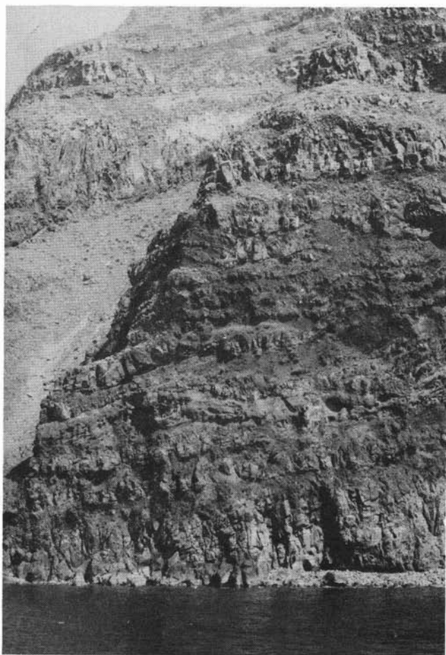
Fig. 1. — Island of Alicudi, western coast. The volcanic sequence attributed to the first cycle of activity on the island, mainly consists of thin lava flows with subordinate interbedded pyroclastic layers.
