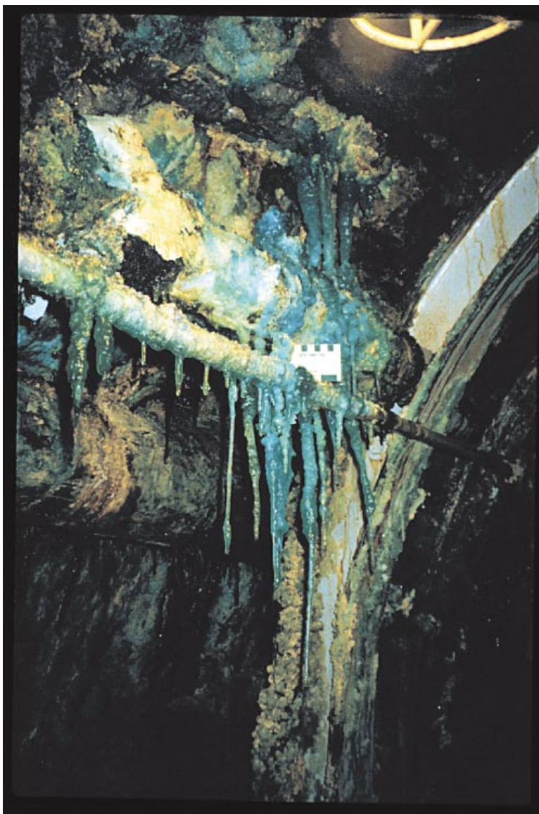
FIG. 2. Stalactites of melanterite hanging from a water pipe in the Richmond adit about 200 m in from the portal and close to where the adit approaches the nearby Mattie deposit.
